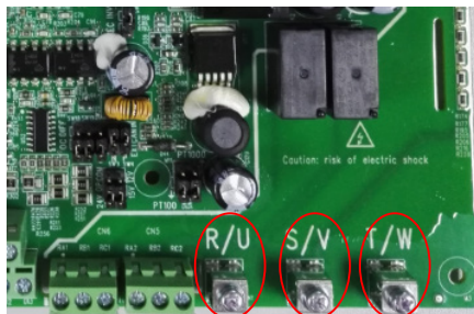
Figure 4-2 Sampling connection of grid phase sequence on control board
